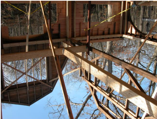
November 2004. Erecting the beams and supports in preparation of adding the second floor and the roof.
