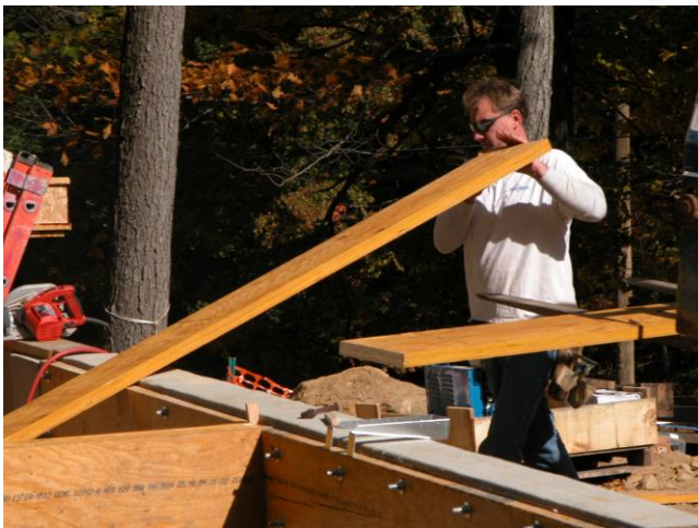
October 2004. Pete Hansen, Project Supervisor lowers joists for the construction of the first floor.
